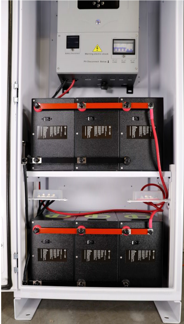
Figure 5.0 – Six Total PHI Batteries are Directly Bussed in Two Sets of Three, then Paralleled Using Cabling to a Single Positive Terminal Block and a Single Negative Terminal Block
